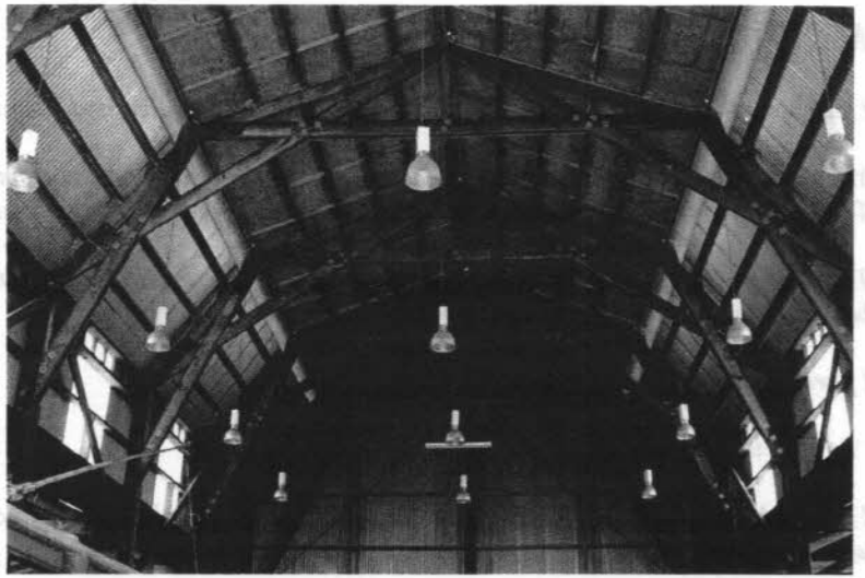
The roof & ceiling structure of the cable car display was constructed in the early 1900's and later transported to the site.
