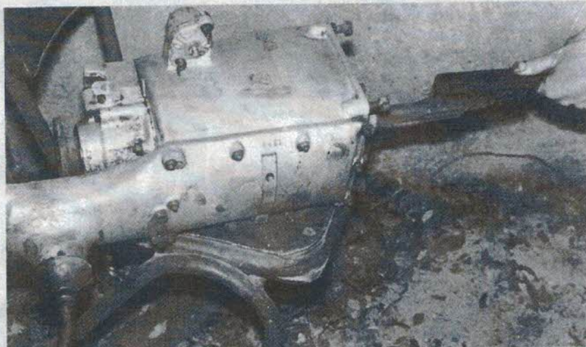
The splines on the replacement gearbox were carefully cleaned to prevent binding.
